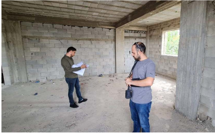
Figure 24. Infill walls made of cement hollow blocks
