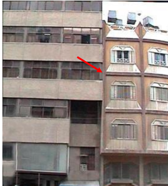
Figure 21. Improper separation between buildings
