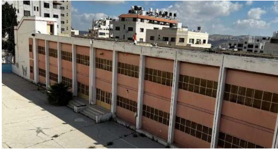
Figure 15. A school building with a regular plan shape and irregular distribution of vertical elements
