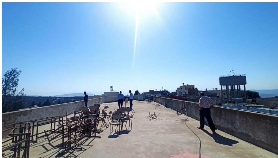
Figure A1: Inspection of roof conditions for a public high school in Yasid – Nablus governorate
