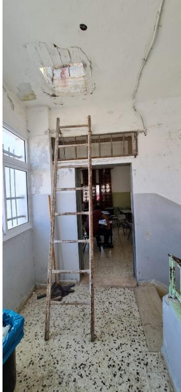
Figure A2: Inspection of structural deficiencies for a public high school in Yasid – Nablus governorate
