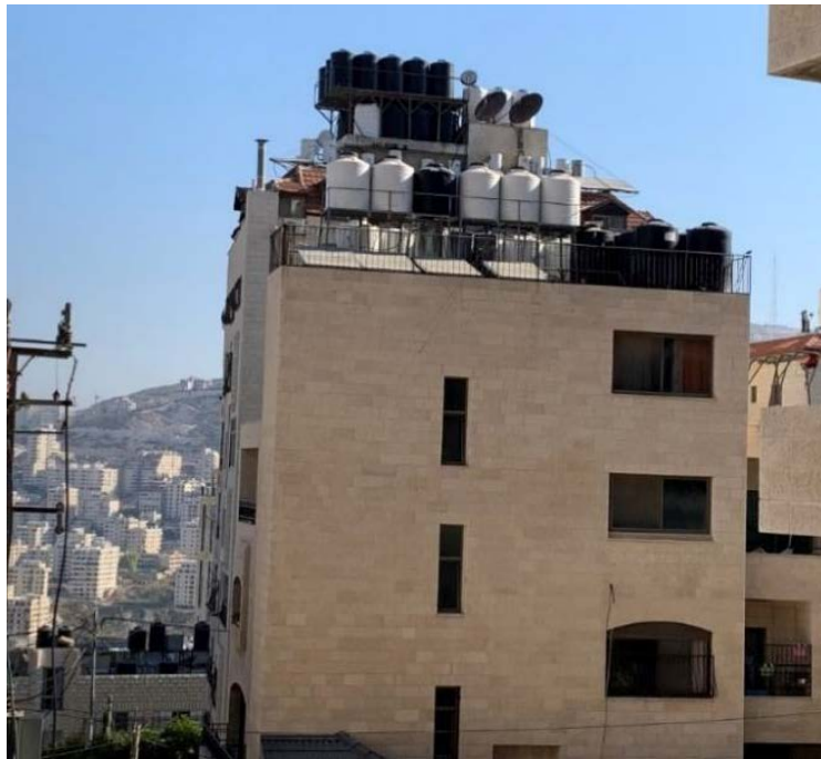
Figure 25. Water tanks installed on the roof of a residential building
