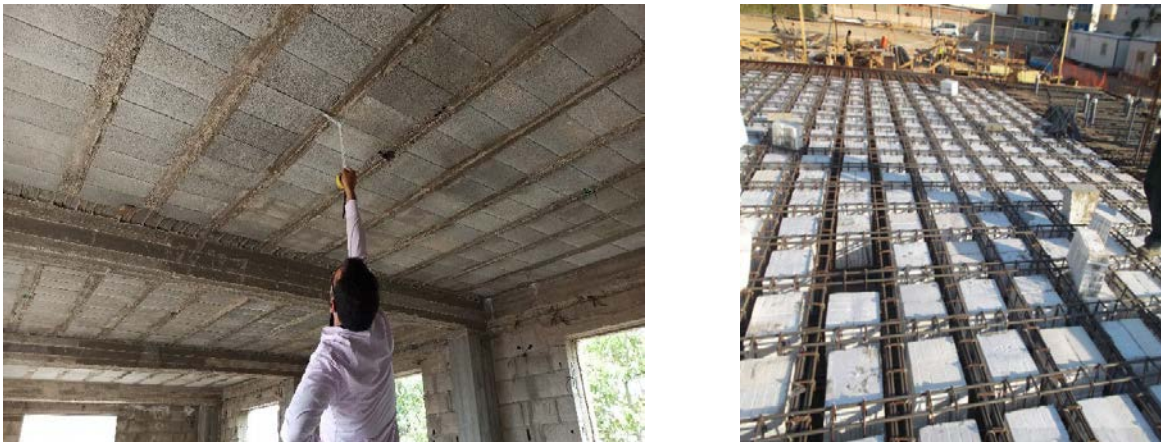
Figure 4. One-way ribbed slab with dropped beams (left) and two-way ribbed slab (right)
